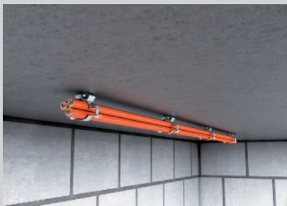
Bundled cable routing under the ceiling.
