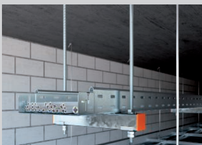
Single-layer ceiling mounting above suspended fire protection ceiling.
