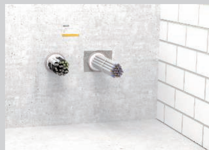
Pipe shells with full assignment with cable bundles and electrical installation pipes.
