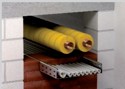
Run-through, non-combustible pipes with section insulation.
