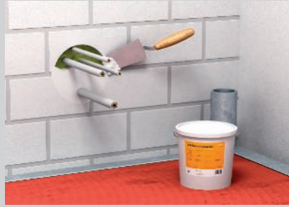
Closure of the surfaces on both sides with the DSX insulation layer creator. (Minimum thickness 1 cm on each side.)
