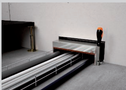
Inserting the box into the wall opening and fastening to the floor
