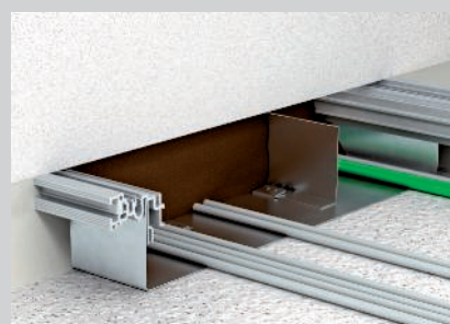
Empty pipes with tension wires can be foamed in for assignment at a later date.
