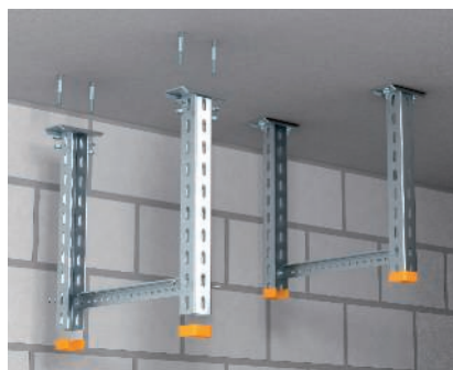
Traverse Mounting of U suspended supports US 3 K, US 5 K and US 7 K under the ceiling using bolt ties and a trapeze, consisting of U profile US 3, US 5 or US 7.
