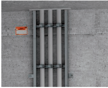
Wall mounting application Wall mounting of a vertical ladder with mounting angles.
