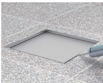
Laying the floor covering on the cassette frames Work the floor covering to the cassette frame. Seal the remaining gap between the floor covering and the cassette frame with suitable materials.
