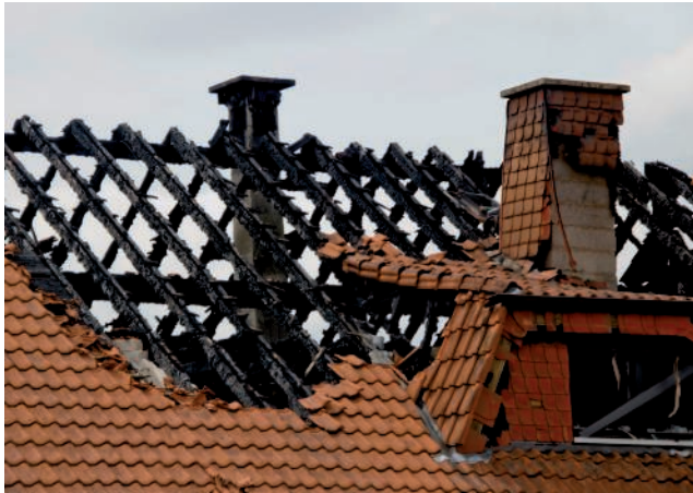
Building damage due to a direct lightning strike
