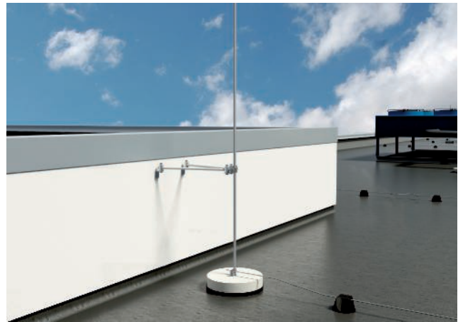
Isolated lightning protection with insulating beams
